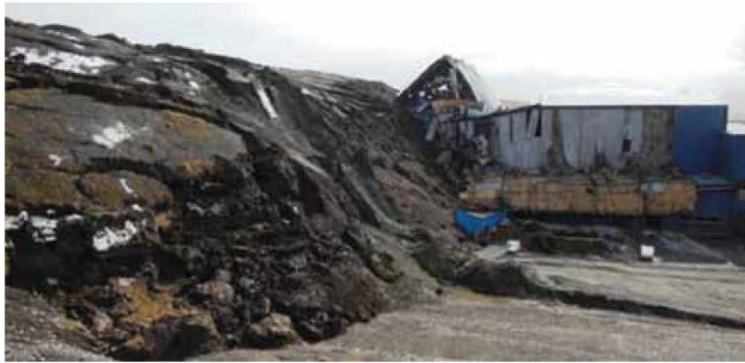
Figure 2: View frontal part of landslide dump in May 2013 that destroyed the administration building and technical service building of the mine
