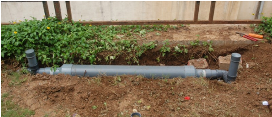
Figure 9: Installed PVC barrel-based sand filter.
